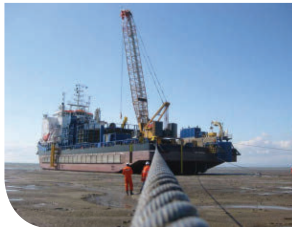
Cable installation for the West of Duddon Sands project in the Irish Sea. Credit: Iberdrola Renewables.
