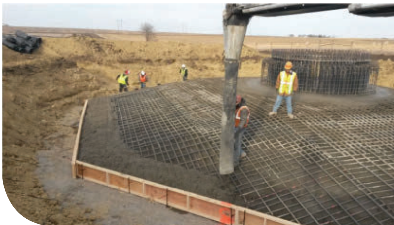
MidAmerican Energy's Highland wind project in O'Brien County, Iowa. Credit: MidAmerican.
